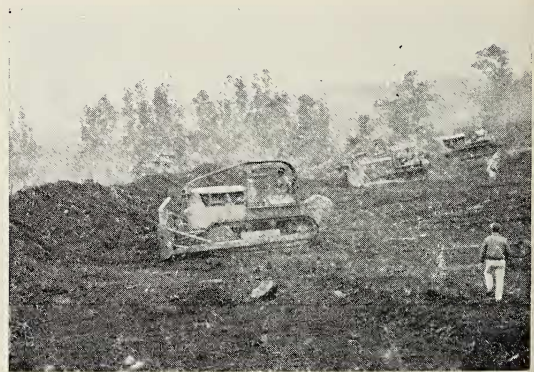
FIG. 5. Bulldozers constructing an earthen barrier in an attempt to keep lava from reaching the Iwasaki camp during the eruption of Kilauea on March 21, 1955.
